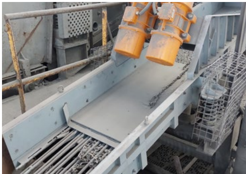
BAR SCREEN CONVEYOR
