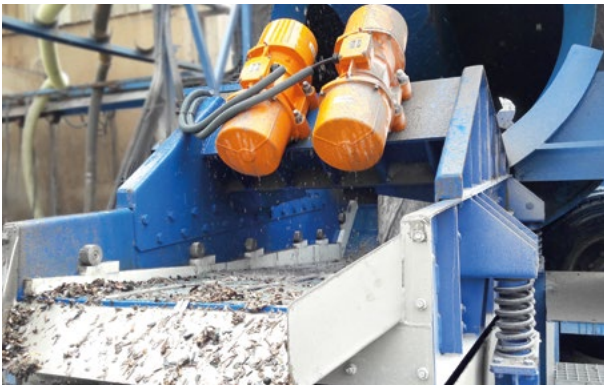
DEWATERING SCREEN AFTER TROMMEL WASHER
