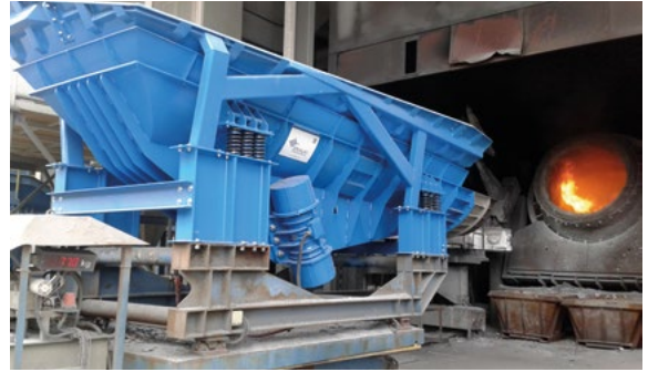
FURNACE CHARGER FOR ROTATORY FURNACE
