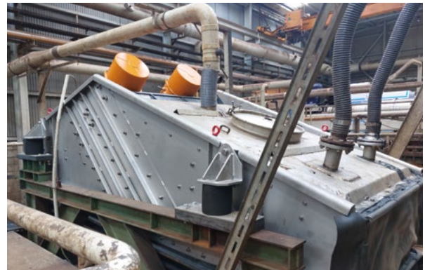
DEWATERING SCREEN IN BIOMETHANISATION PLANT
